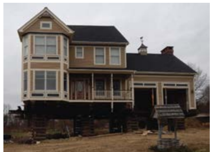
Fig. 2: Replacement of residential foundation in Connecticut (photo courtesy of U.S. Government Accountability Office)
