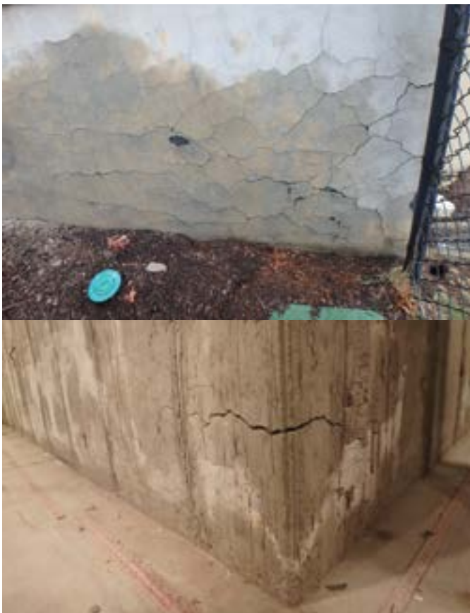
Fig. 1: Typical indications of pyrrhotite deterioration in concrete foundations
